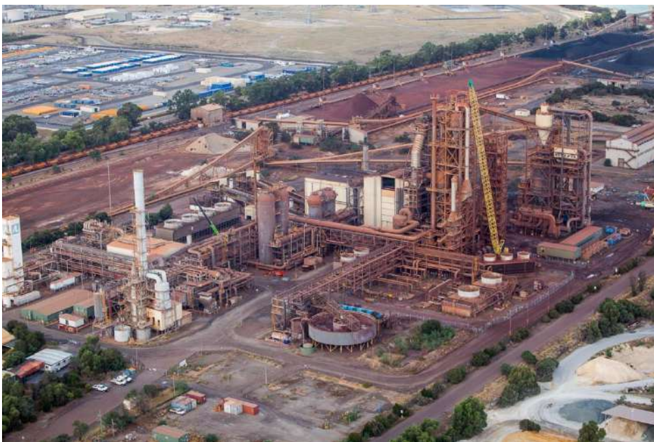
RIO TINTO HiSMELT FACILITY
